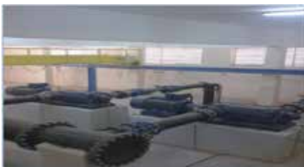
Pumps for AL-Sabein Collection and Storage Project- Sana'a
