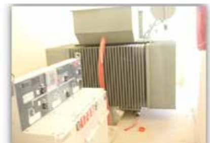
Electric Transformers For AL-Sabein Collection and Storage project -Sana'a
