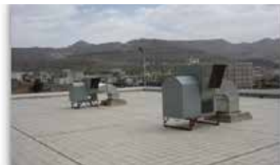
Central air-conditioning for the Central Veterinary Laboratory Building
