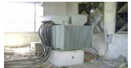
Electric Transformers For Educational Instruments Center Building Project
