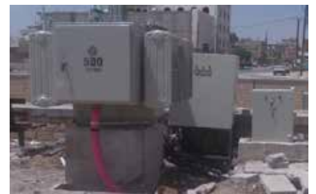
Electric Transformers for North Alsayla project
