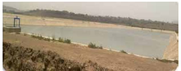
Extension of existing the wastewater treatment facilities at Dhamar water supply system project - Dhamar city.
