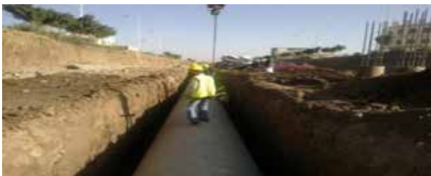
Main GRP Pipeline (1400 mm)
